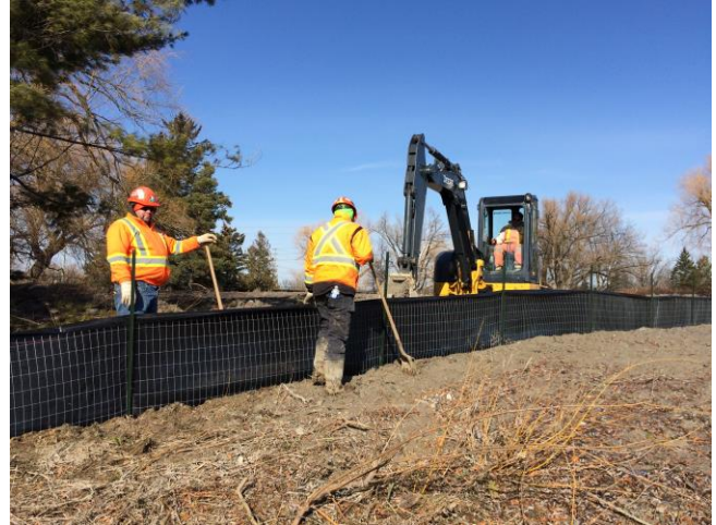
February 27, 2018. Installation of Environmental Controls, south of Rutherford Rd. Steel-mesh fence controls sediment flow from preloading sites.
